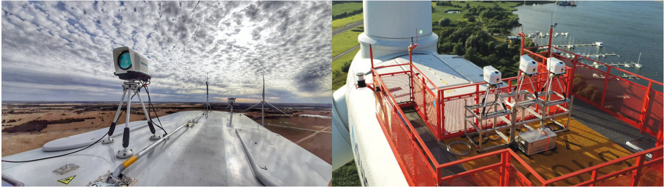
Fig. 1 Photo of WCN installation (left: WCN on onshore WTG, right: WCN on offshore WTG)
